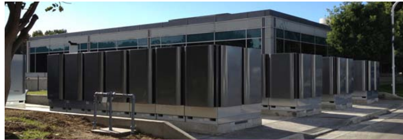
A new stationary fuel cell system installed in March 2013 on the Torrance, Calif., campus of American Honda will produce one megawatt of clean, low-CO 2 energy.
